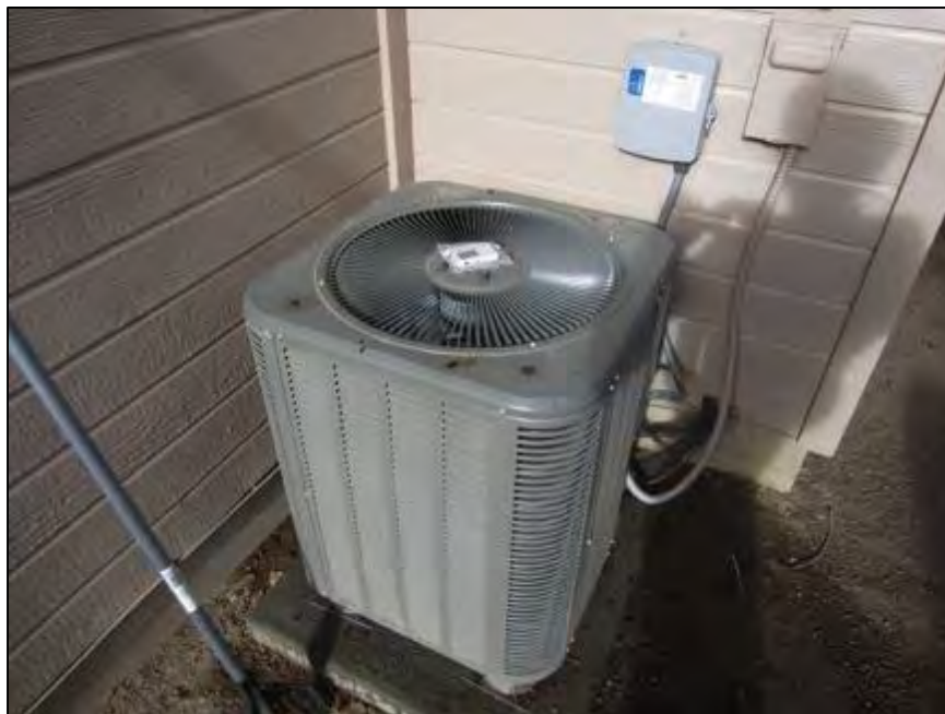
Figure 28. Motor Logger on Condenser
