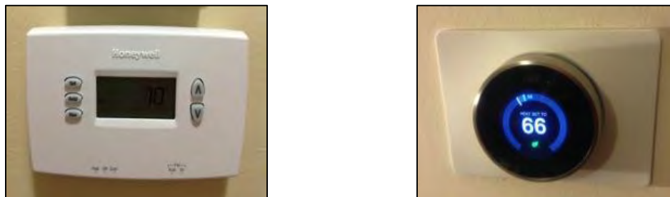
Figure 2. Programmable (left) and Nest (right) Thermostats Installed in Program Participant Homes
